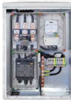
Measuring transformer 500 / 5 A
